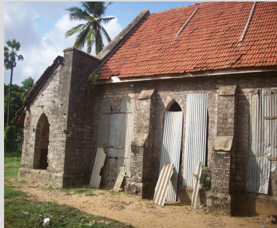
Rear of the damaged St. Andrew' s Pallai
